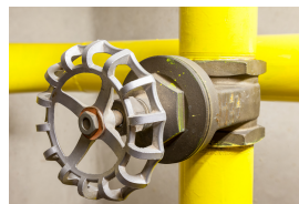
Master shut-off gate valve
